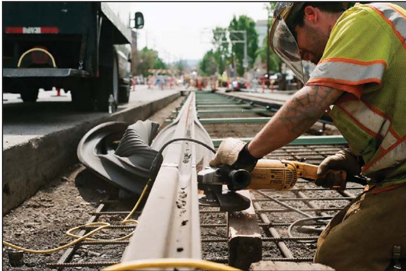
Crews installed the rubber insulation on the new trackway in Portland's Lloyd District as part of the Streetcar Loop Project.
