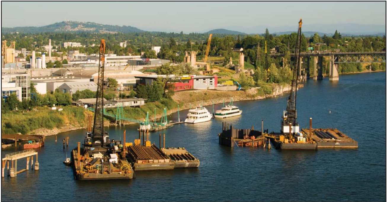
In-water construction of the new Portland-Milwaukie Light Rail Bridge started on July 1, 2011.
