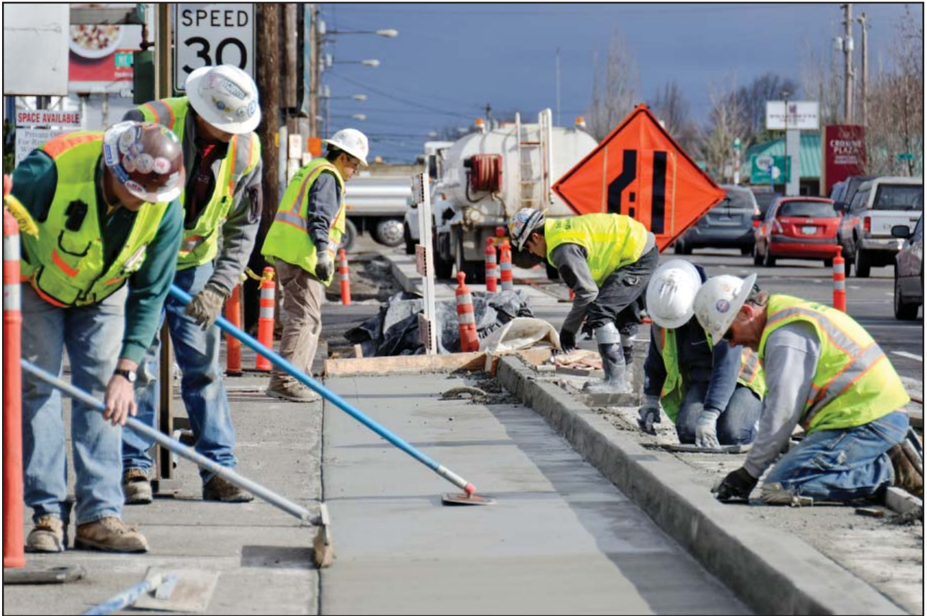
Crews extended the sidewalk on N Weidler Street as part of Portland Streetcar Loop construction.
